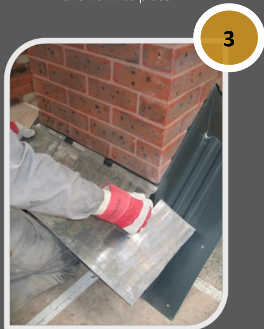
Trim lead to size and cut out notches where mortar lines fall
